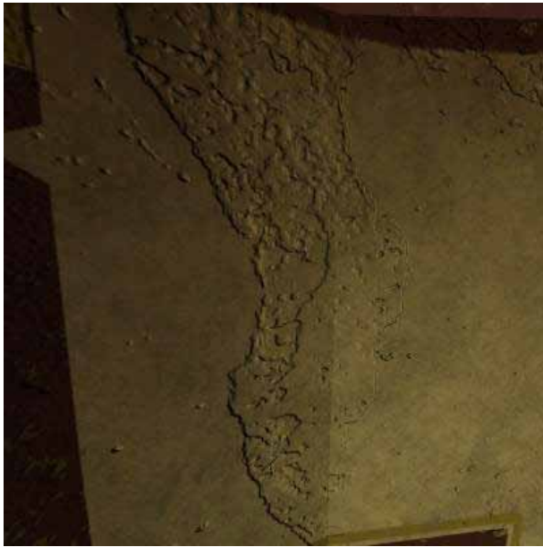
Figure 11: A digital rendering of wall cracks in the small East Church
