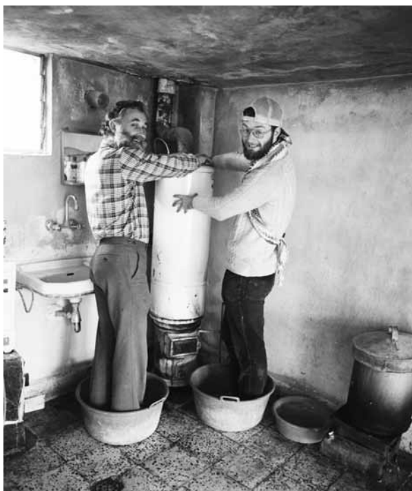
Figure: 9 Ian Edwards and Stephen Bourke at Pella 1985 repairing a hot water service. Image: courtesy Stephen Bourke.
